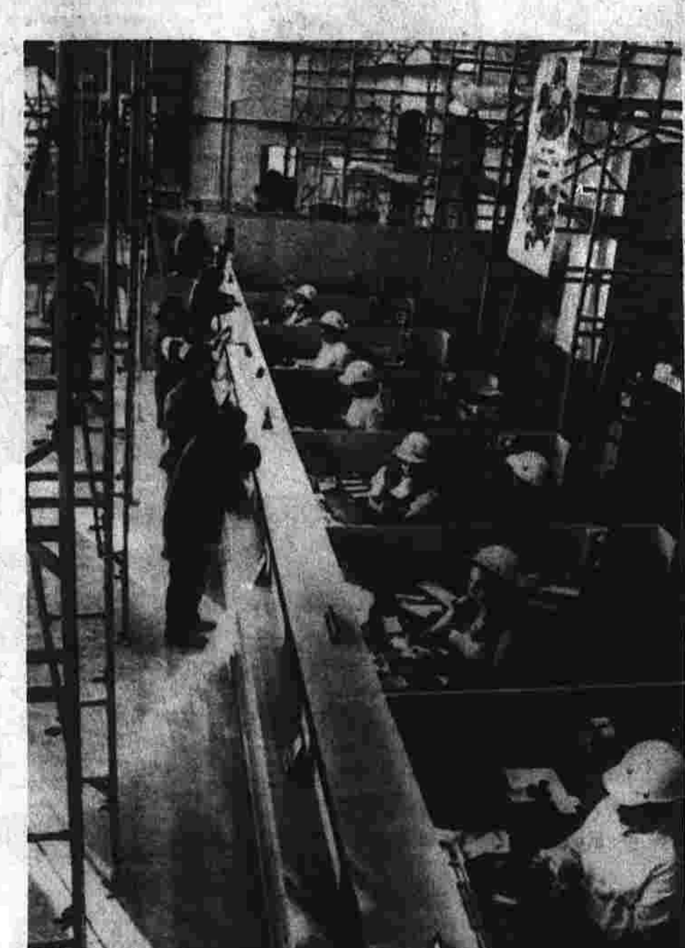
Bank tellers wear hard hats to work under scaffolding at the Merchants National Bank in New Bedford, Mass., while a renovation project is under way.
